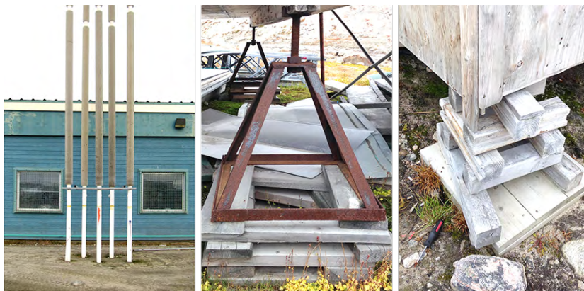
Foundation from left to right: thermo-syphon, steel footing under wood beam, adjustable wood cribs. Courtesy of the author.
